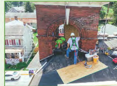
Left: Installing a stealth cell antenna to an existing bell tower, maintaining the historic look of the building while replacing the bell with steel structure for mounting antennas in Glen Rock, PA. (Photo: ECI Wireless)
