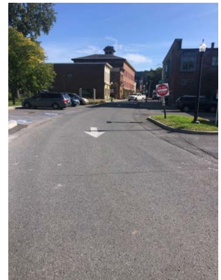
Betke Blvd lacking bike/ped facilities
