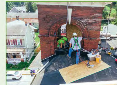
Left: Installing a stealth cell antenna to an existing bell tower, maintaining the historic look of the building while replacing the bell with steel structure for mounting antennas in Glen Rock, PA. (Photo: ECI Wireless)
