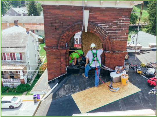
Right: Installing a stealth cell antenna to an existing bell tower, maintaining the historic look of the building while replacing the bell with steel structure for mounting antennas in Glen Rock, PA. (Photo: ECI Wireless)
